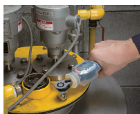
Safe to work around water.
